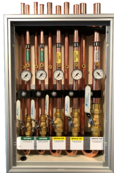
Shown above VZU22334 - 5 valve box are shown with gauges, NFPA gas identification and flow arrows applied.
